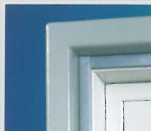
Fire Seal around Door
